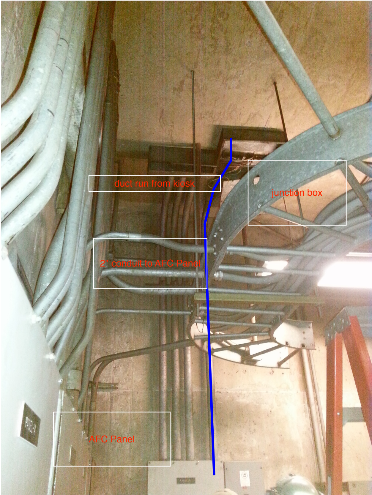
Photo #2 – G03 Addison Road: Junction box to AFC Panel
