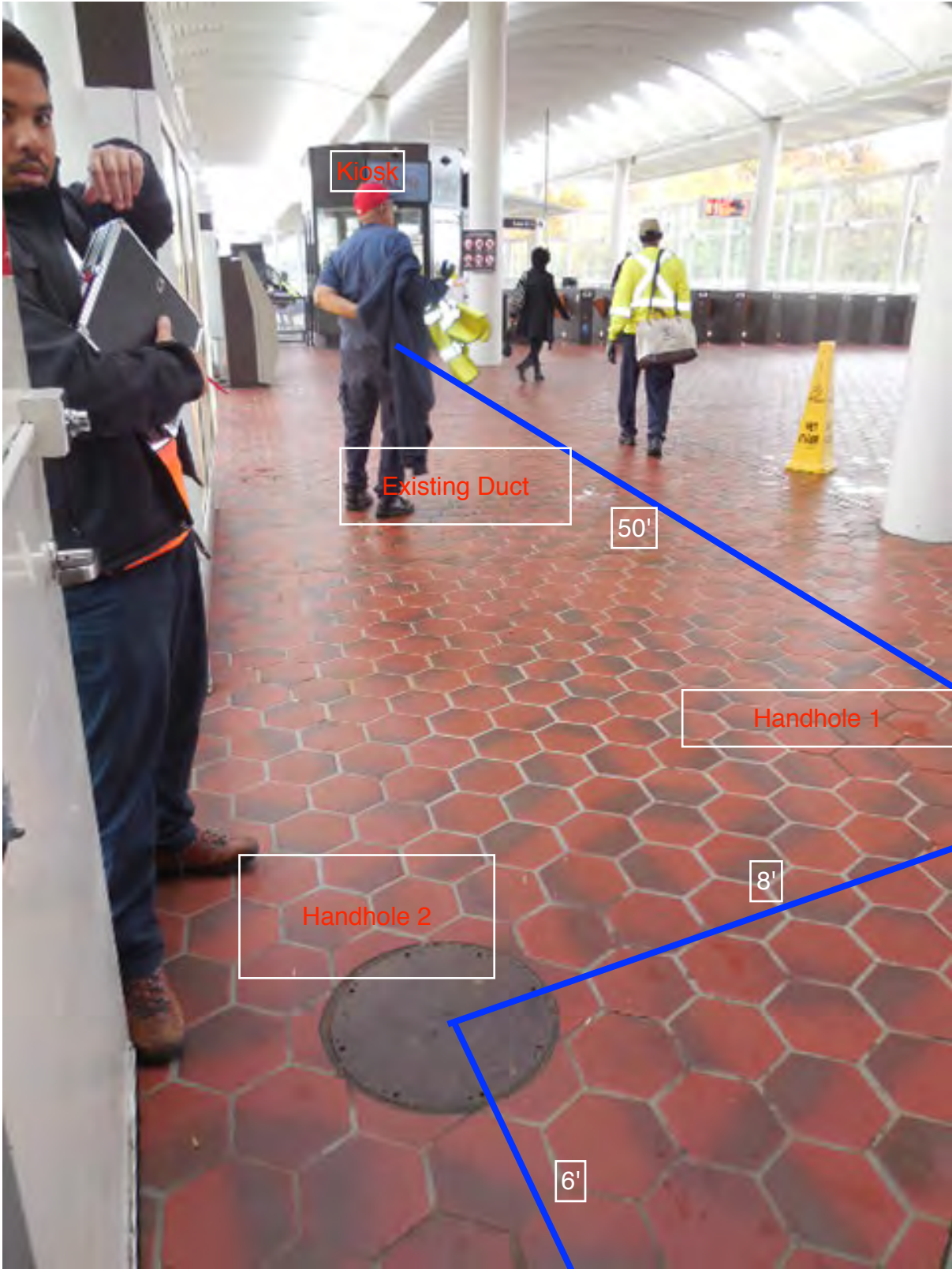
Photo#1 – Existing duct layout on mezzanine floor
